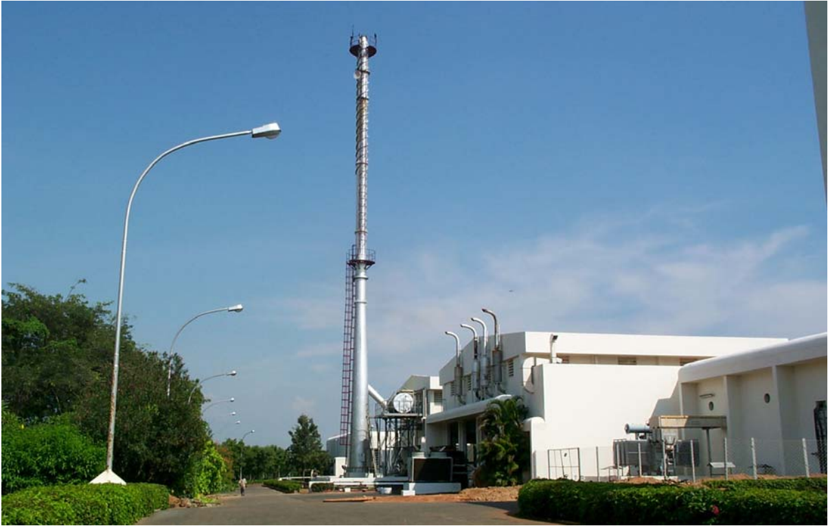
PHOTO 1: EXISTING OIL FIRED BOILER
