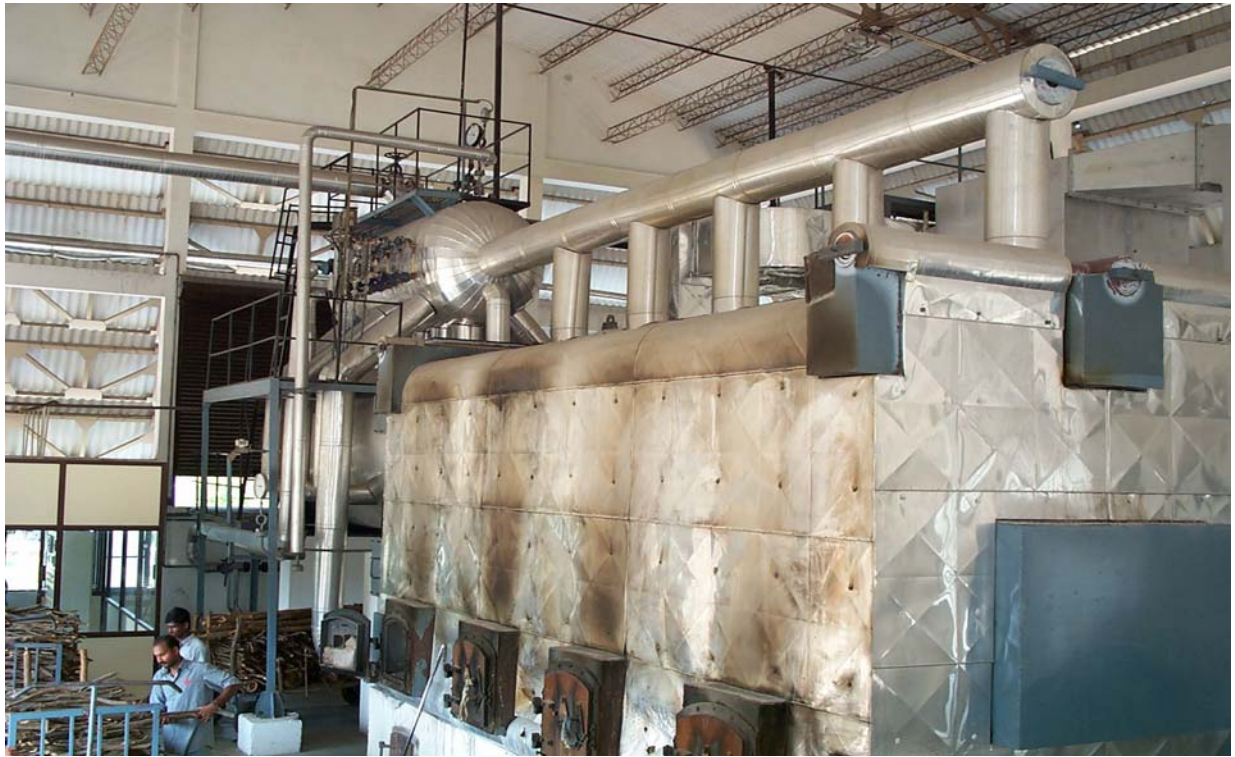
PHOTO 3: PHOTOGRAPH SHOWING THE BOILER FURNACE, SHELL & STEAM DRUM
