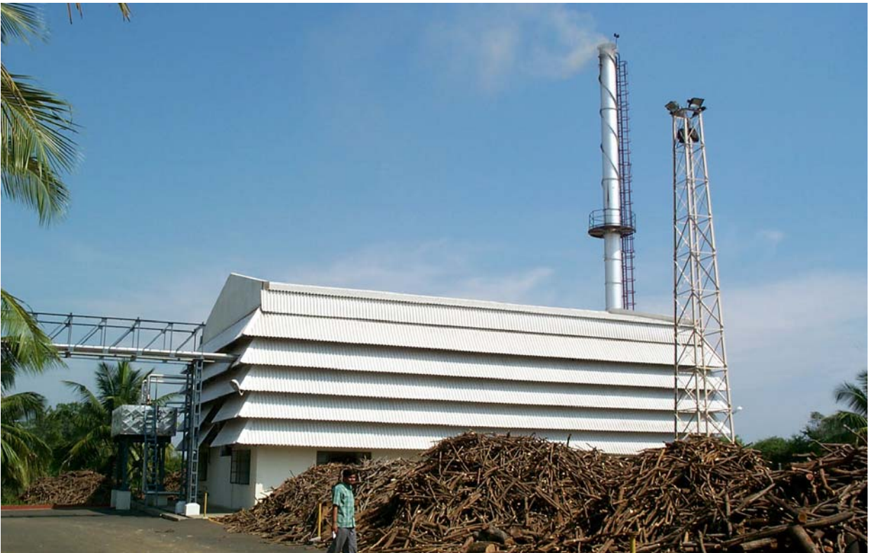
PHOTO 2: NEW WOOD FIRED BOILER
