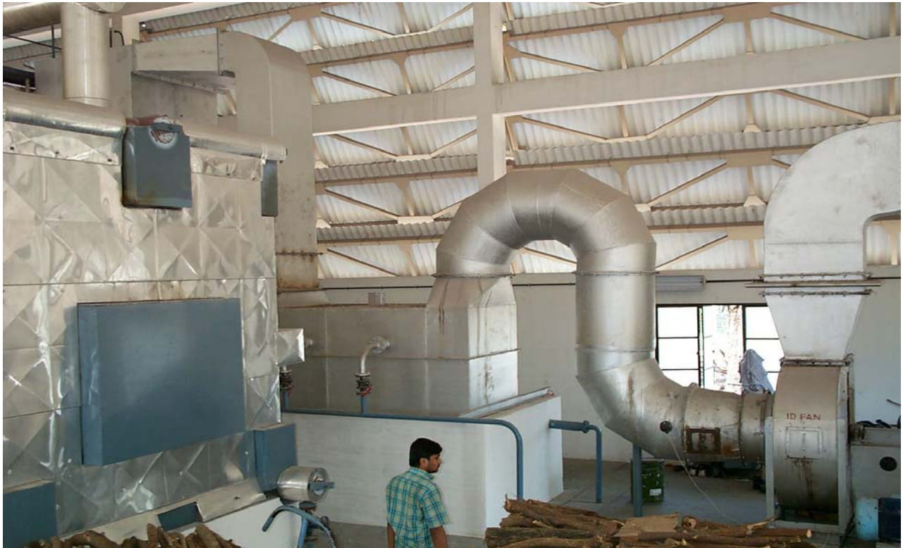
PHOTO 4: PHOTOGRAPH SHOWING THE WET BOTTOM DUST TRAP
